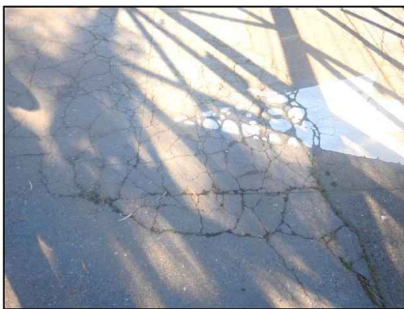
Cracked, deteriorated asphalt
