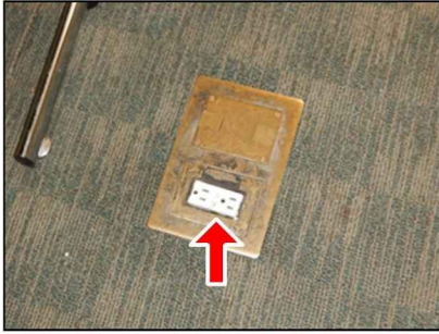
Improper floor receptacle
