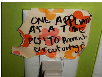
Sign indicating overloading
