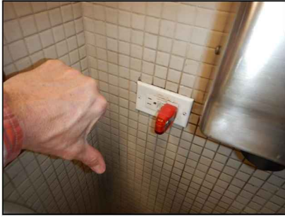
Defective GFCI receptacle
