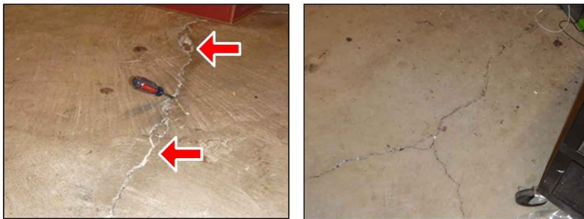
Cracking in slab
