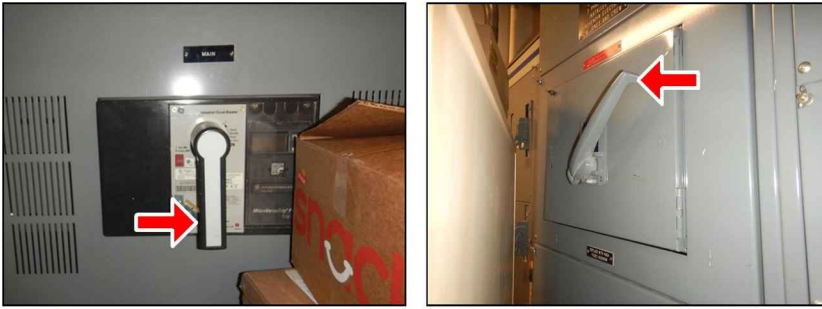
Main electrical disconnects
