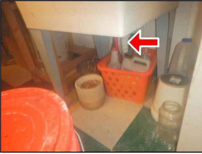
Missing utility sink leg
