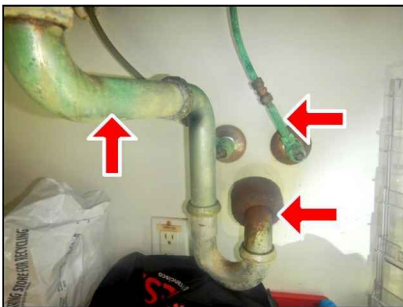
Surface corrosion below sink
