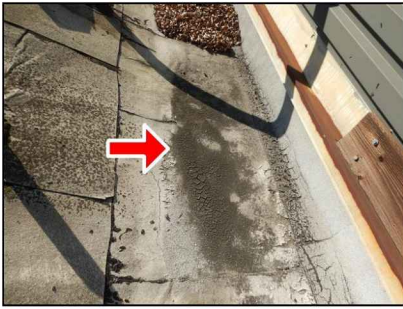
Evidence of ponding
