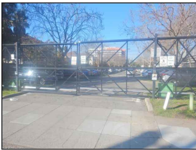
Automatic gates not tested
