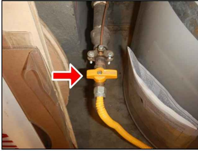
Gas valve closed
