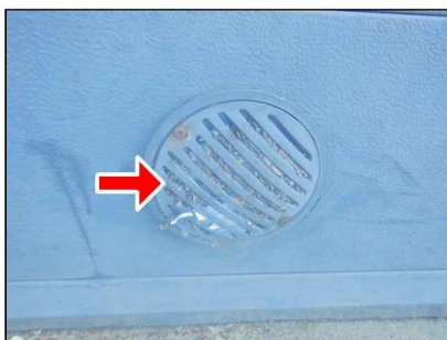
Clogged roof drainage outlet
